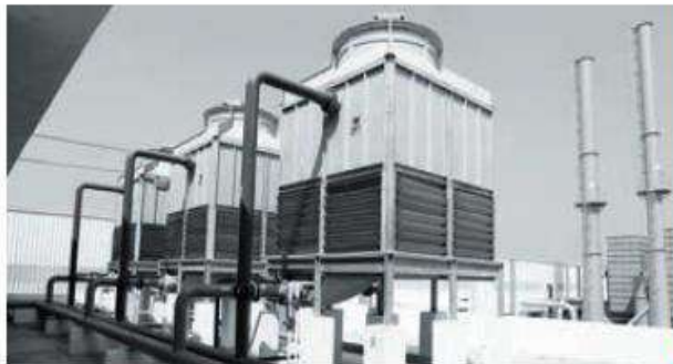
Chilling plant cooling towers New plant at Hunegundepalle village
